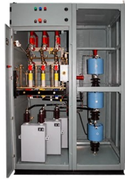
APFC Relay Panels (Thyristorised & Conventional)
