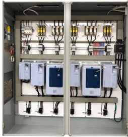
AC & DC Drive Control Panel
